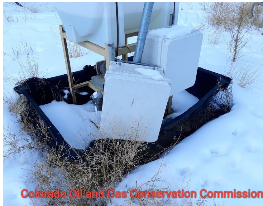
Photo 2 Bird netting in disrepair.
