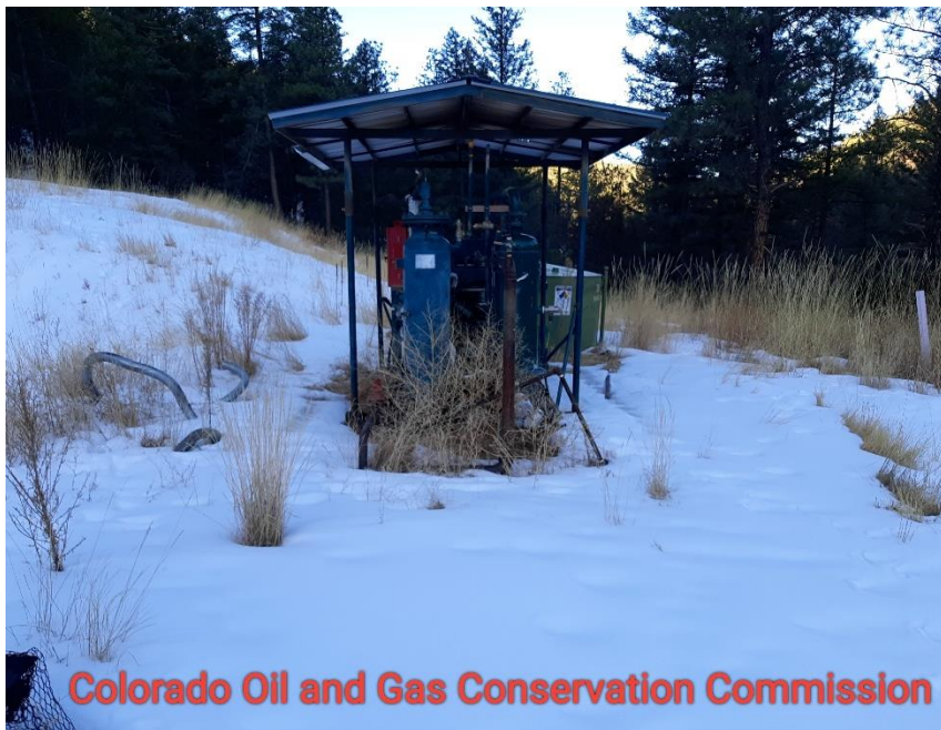
Photo 3 Dead weeds around compressor
