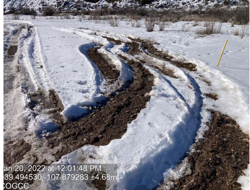
Lack of stabilization/compaction
