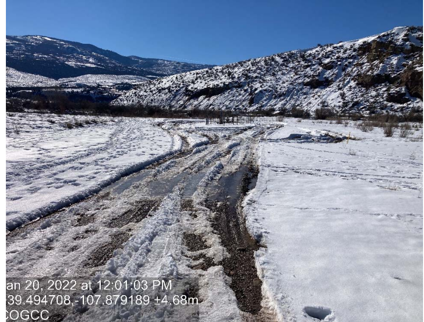
Lack of stabilization/compaction
