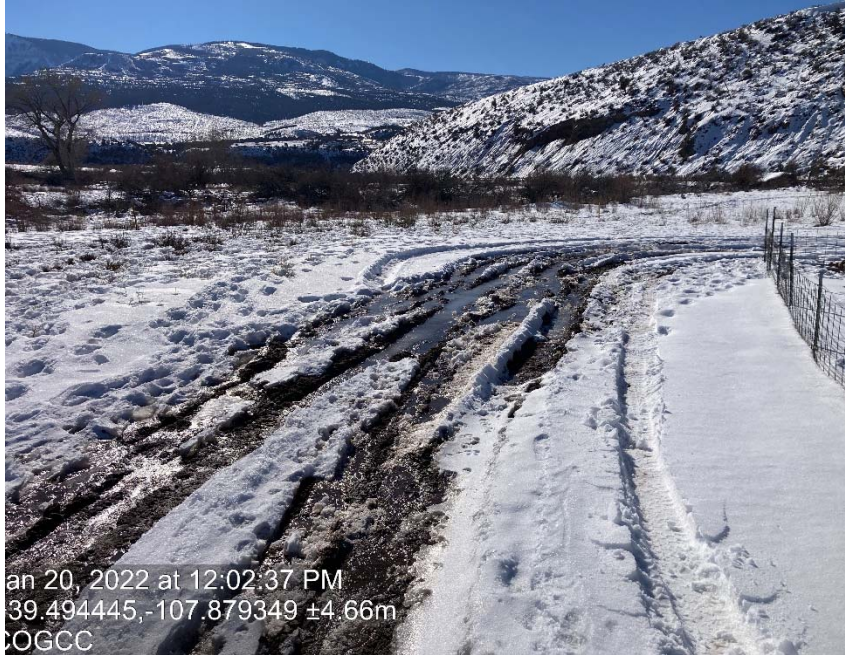
Lack of stabilization/compaction
