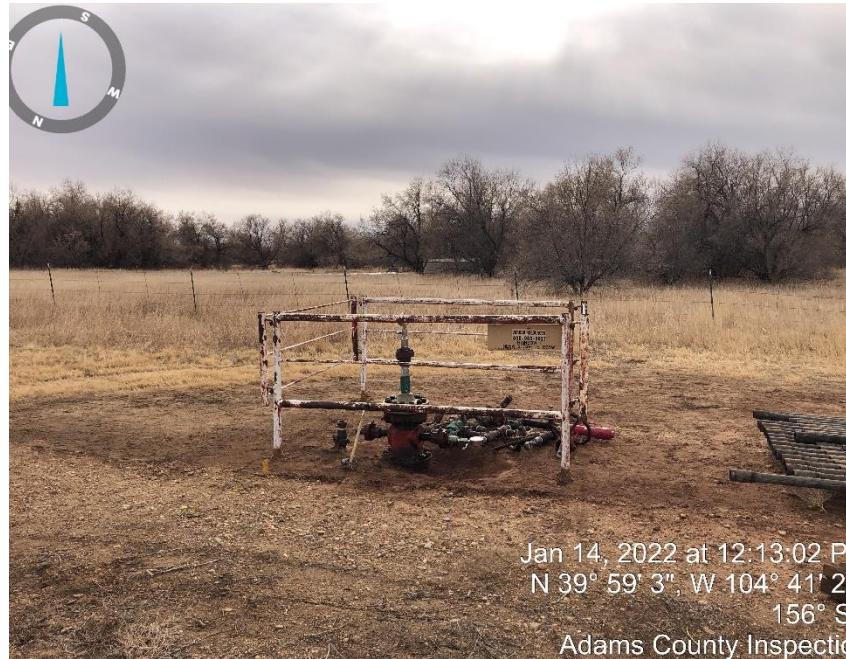
Photo #3 Well Head.
