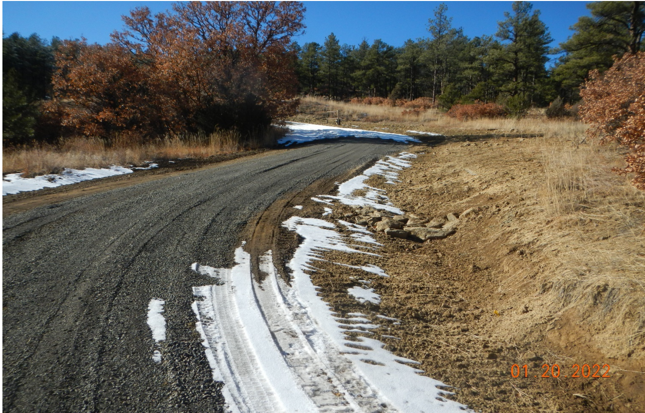
Photo 3. Facing southwest toward the access road near the location. The disturbance area has been reclaimed and gravel was spread along this area of the road. Check dam has been repaired.
