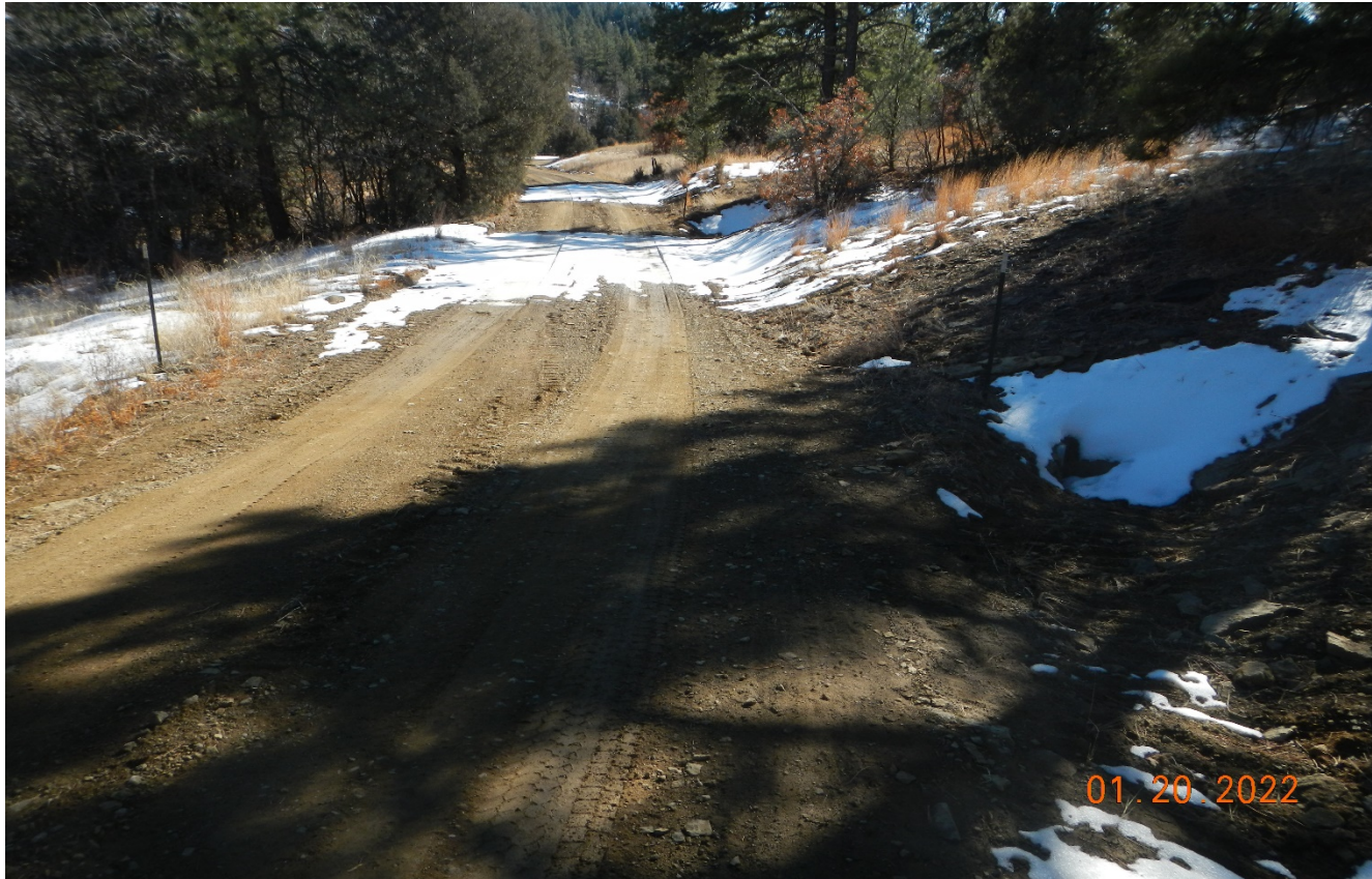
Photo 1. Facing southeast along the access road. The culvert along the road have been repaired.
