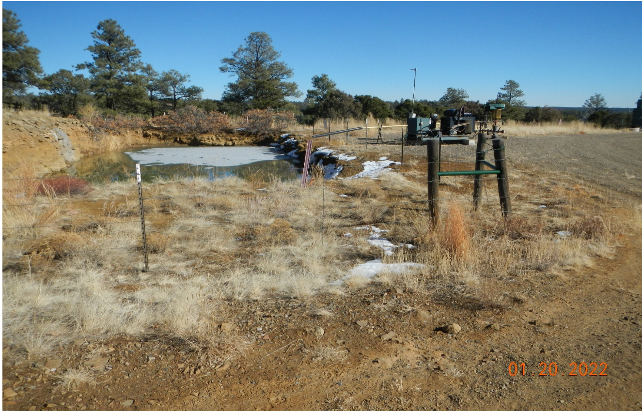
Photo 1. Facing east toward the well site. The fence has been repaired around the pit and an extension pipe was added to the PW discharge.
