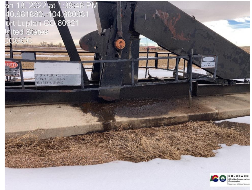
Pic 2 leaking gear box, stained soil needs to be cleaned up, oil on cement needs to be cleaned up.
