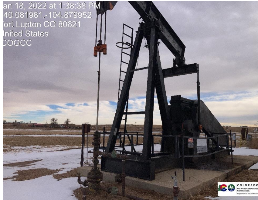
Pic 1 Wellhead, pump jack.
