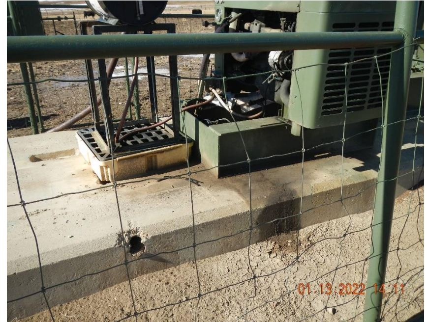
Staining beneath prime mover.
