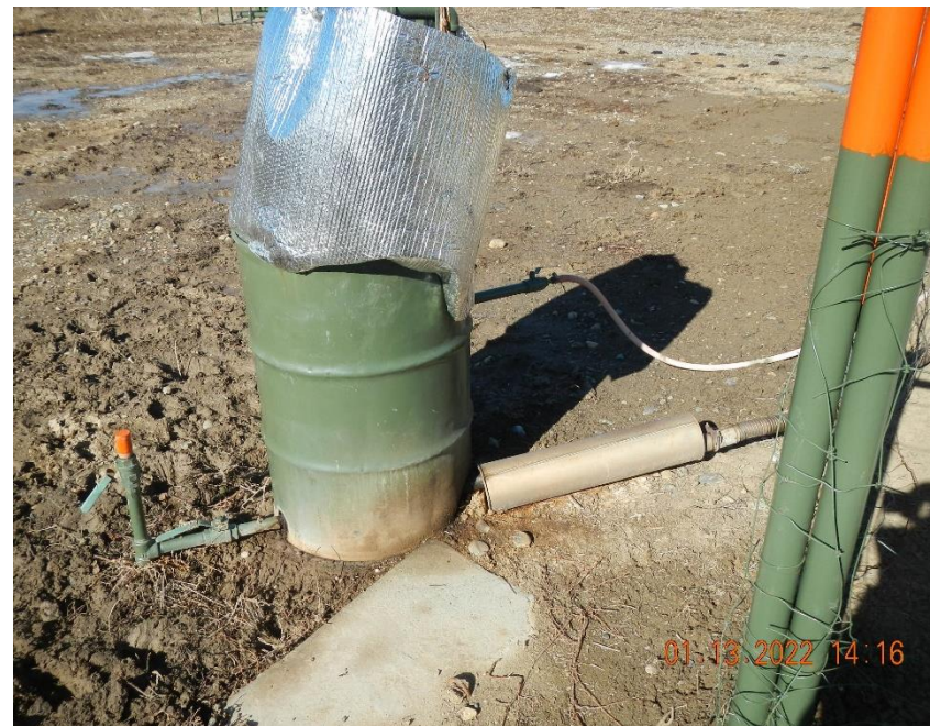
Drop out tank for supply gas. Prime mover exhaust ported into drum.
