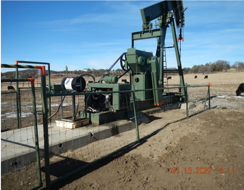
Staining beneath the prime mover on the concrete pad and adjacent soil.
