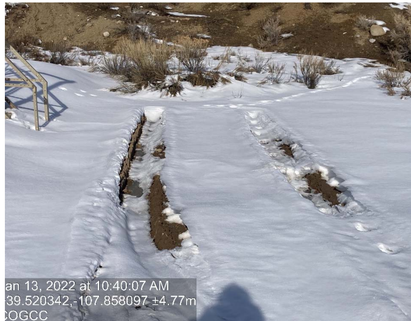
Lack of stabilization/compaction
