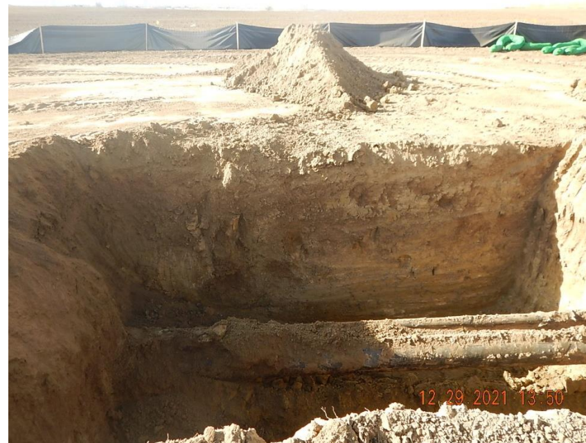
View of flowlines exposed in excavation at Firecracker release: (1) 10" carbon steel Firecracker consolidation flowline; (1) 2" carbon steel off location gas flowline.
