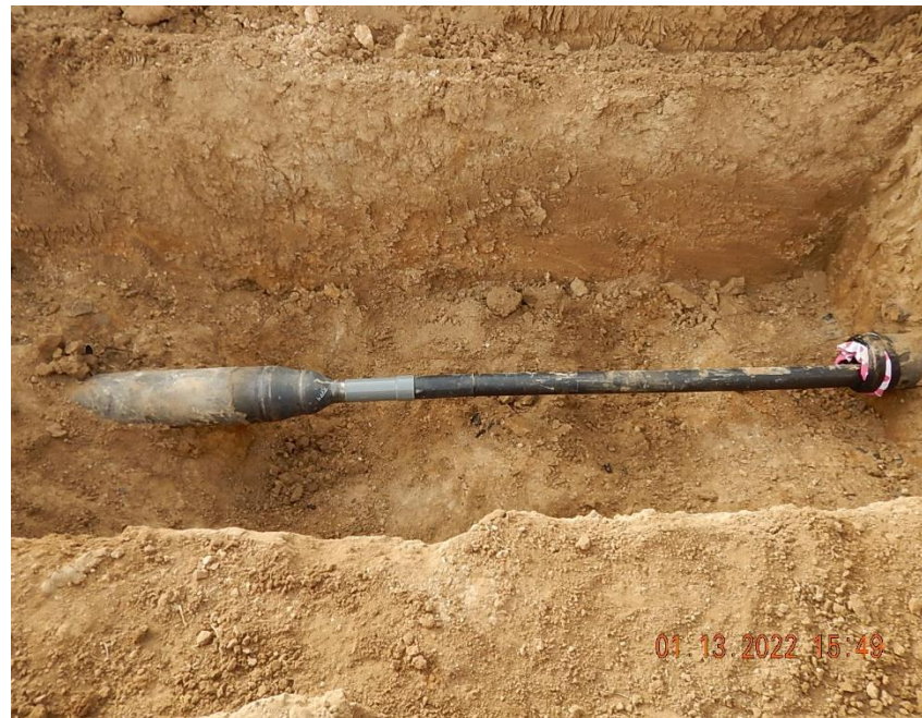
Flowline repairs being completed at south bell hole excavation. 10" OD CS pipe to 4" OD HDPE pipe transition. Approximately 1245' linear feet of 4" HDPE pipe sliplined through existing 10" firecracker consolidation flowline (across failure point at spill ID #481413).
