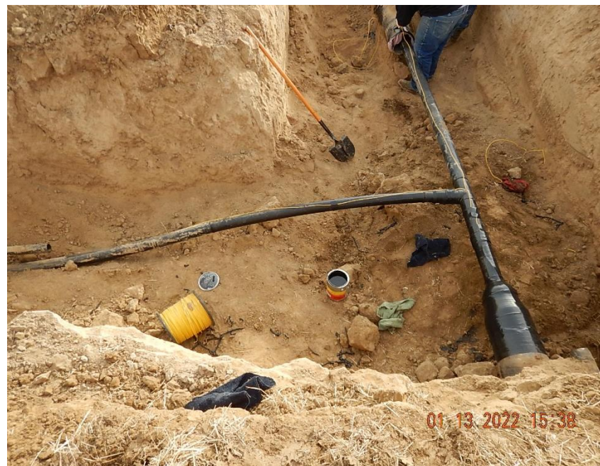
Flowline repairs being completed in north bell hole excavation. 10" CS pipe to 4" HDPE pipe transition; 3" HDPE flowline tie in from Foreman Unit #2 well. Tracer wire being installed at time of inspection.
