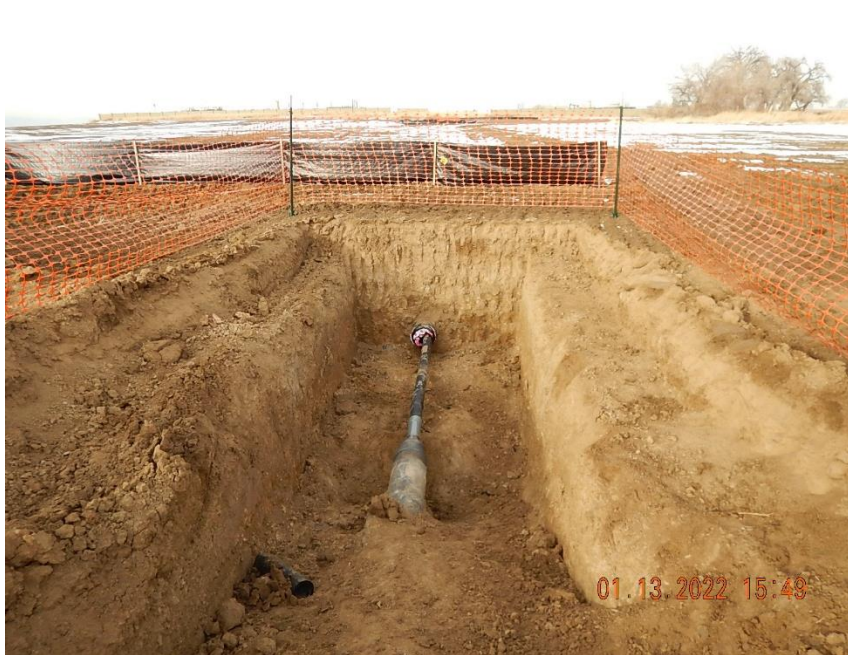
View from south bell hole excavation to north toward the Firecracker release point; flowline repairs in progress.
