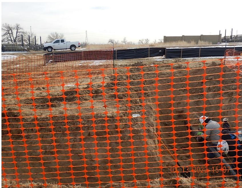
View from north bell hole excavation to south toward the Firecracker release point; KPK field personnel in process of completing flowline repairs.
