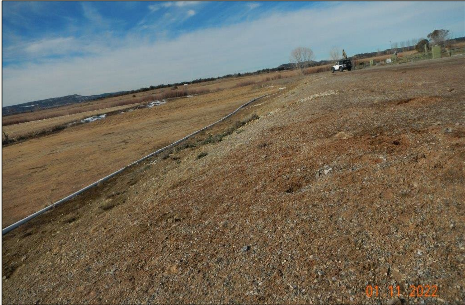
Photo 2. View of the southern fill slope from the southeastern corner facing westward. Revegetation appears to be progressing, largely in a grazed vegetative condition at this time, needs to be assessed during the active growing season.
