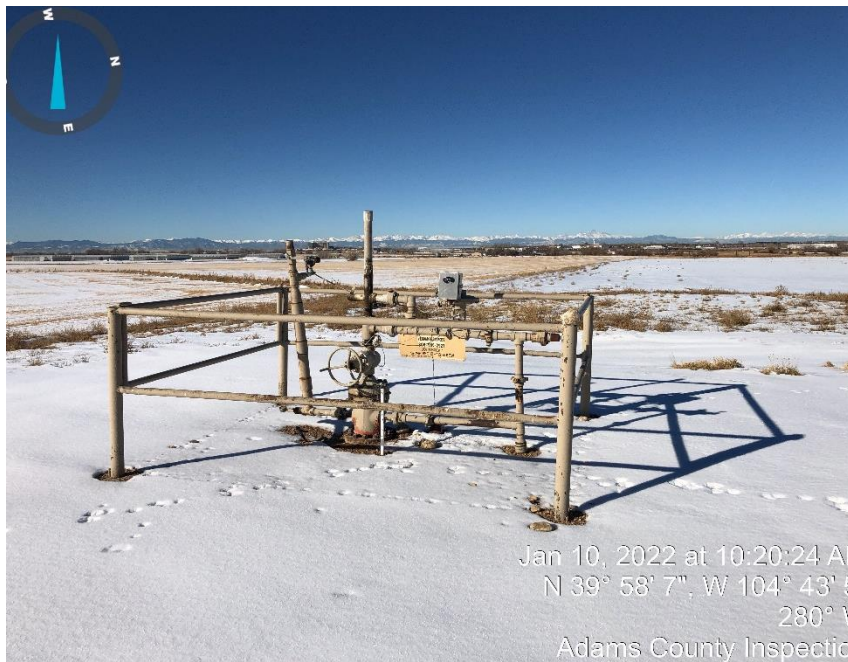
Photo #3 Well Head.
