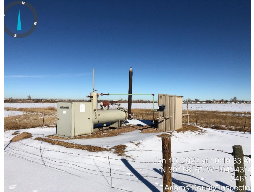
Photo #2 Meter & Separator.
