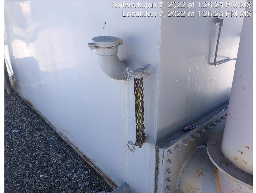
Photo #5632 Sight glass indicates the storage tank is full of an unknown fluid.
