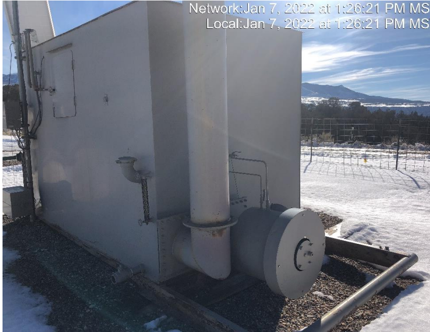
Photo #5631 Storage tank not labeled.
