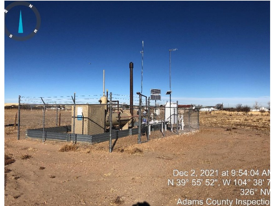
Photo #2 Meter & Separator.
