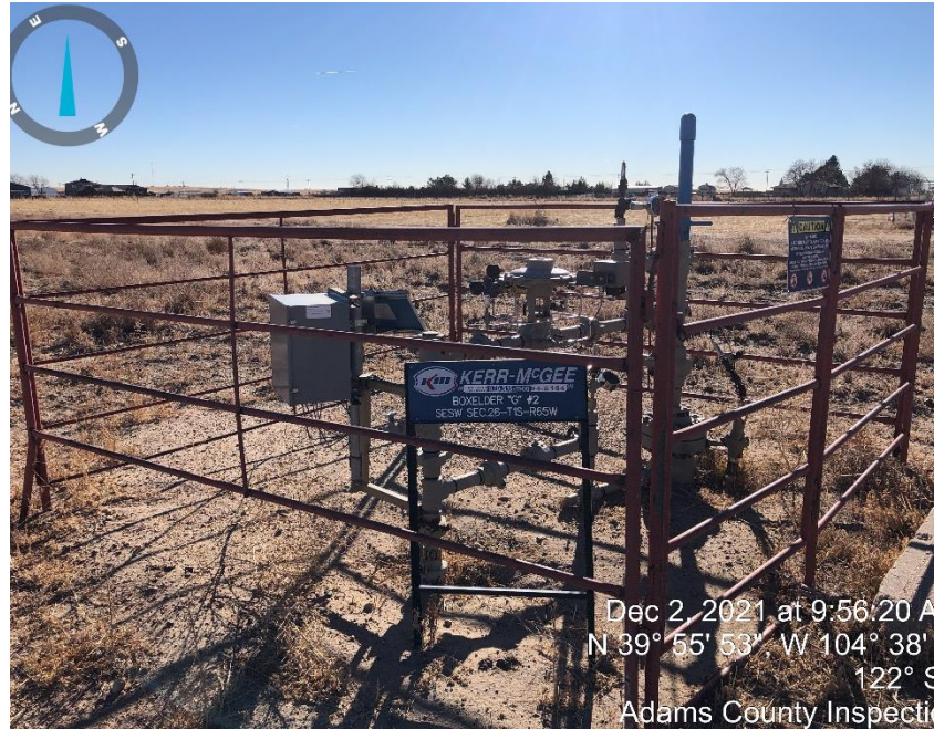
Photo #3 Well Head.
