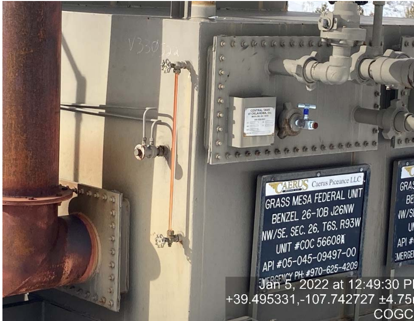
Storage tank sight glass shows fluid in it
