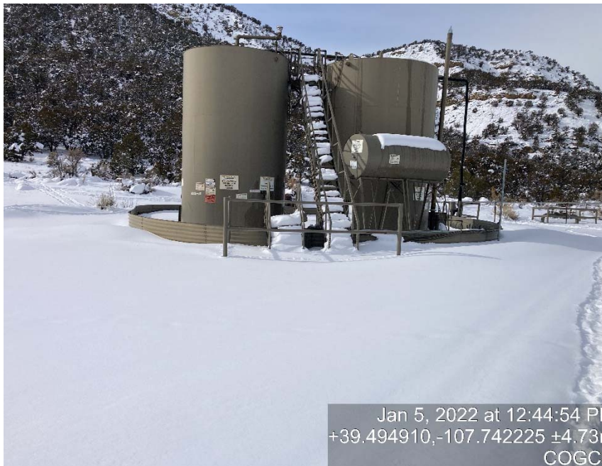
Location/lack of battery signage
