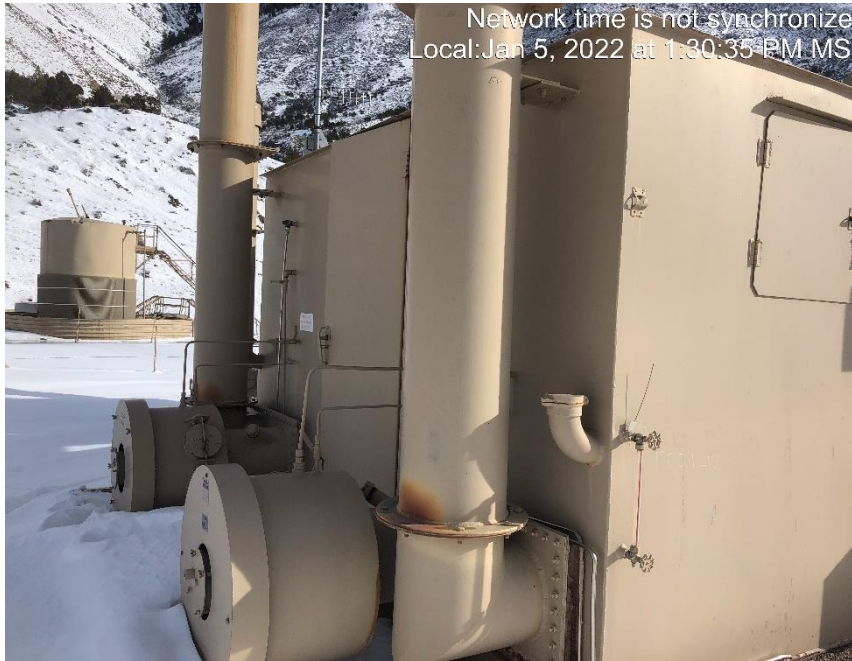
Photo #5597 Storage tank not labeled.
