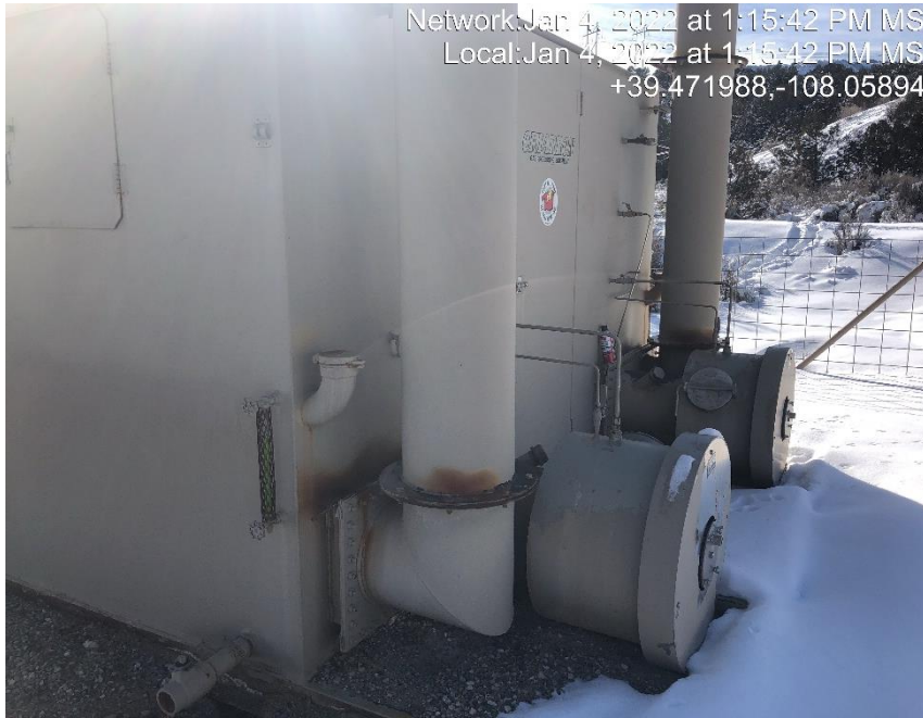
Photo #5575 Storage tank not labeled.
