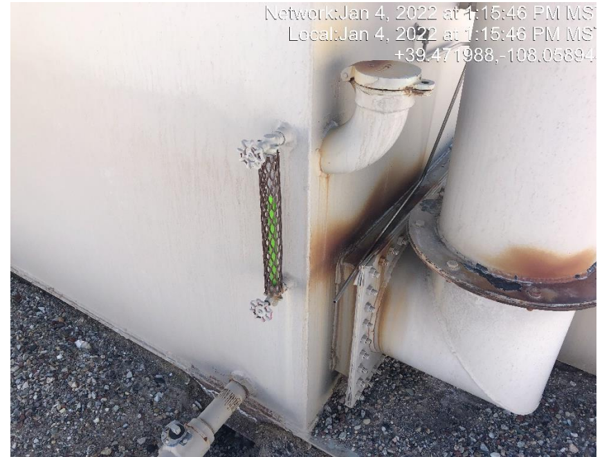
Photo #5576 Sight glass indicates the storage tank is full of an unknown fluid.
