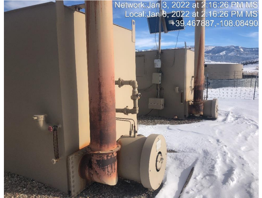
Photo #5564 Storage tanks not labeled.
