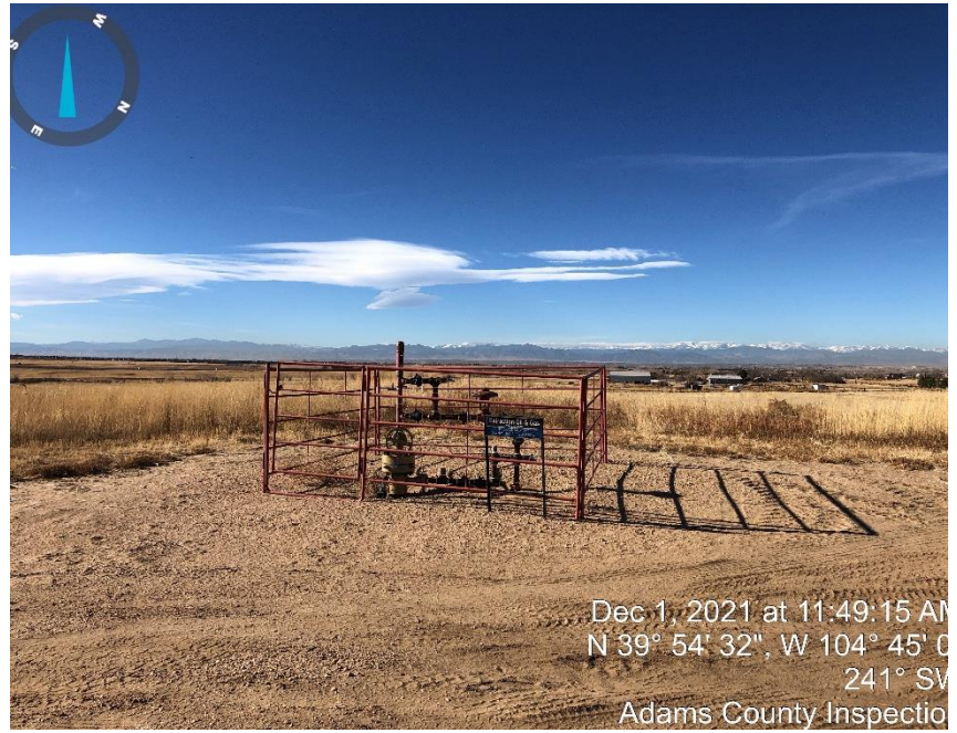
Photo #3 Well Head.
