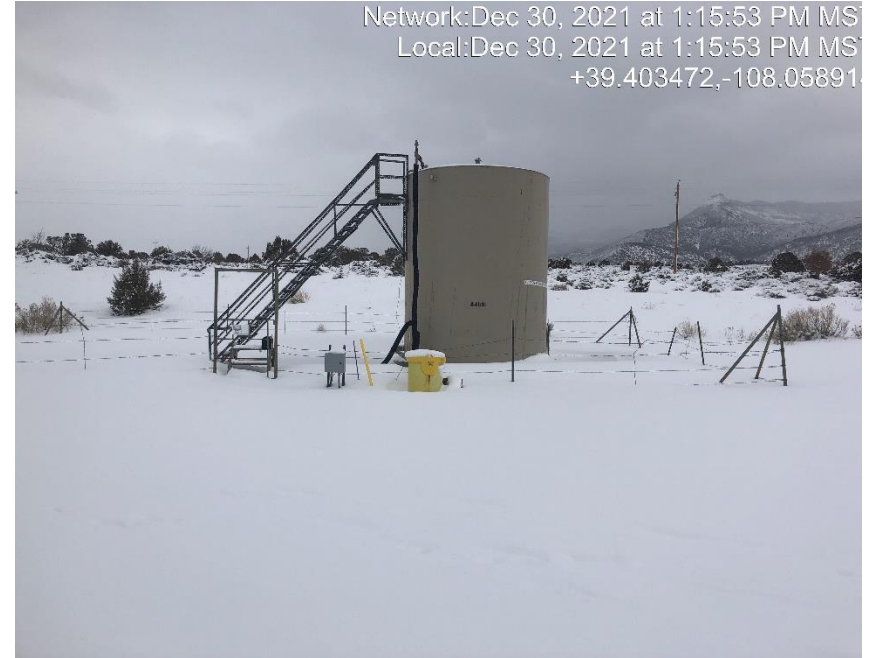
Photo #5546 No battery sign located at the tank battery.
