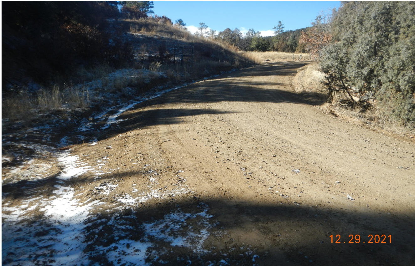
Photo 4. Facing along the access road near the location. The area of erosion was repaired and drainage s directed toward the culvert.
