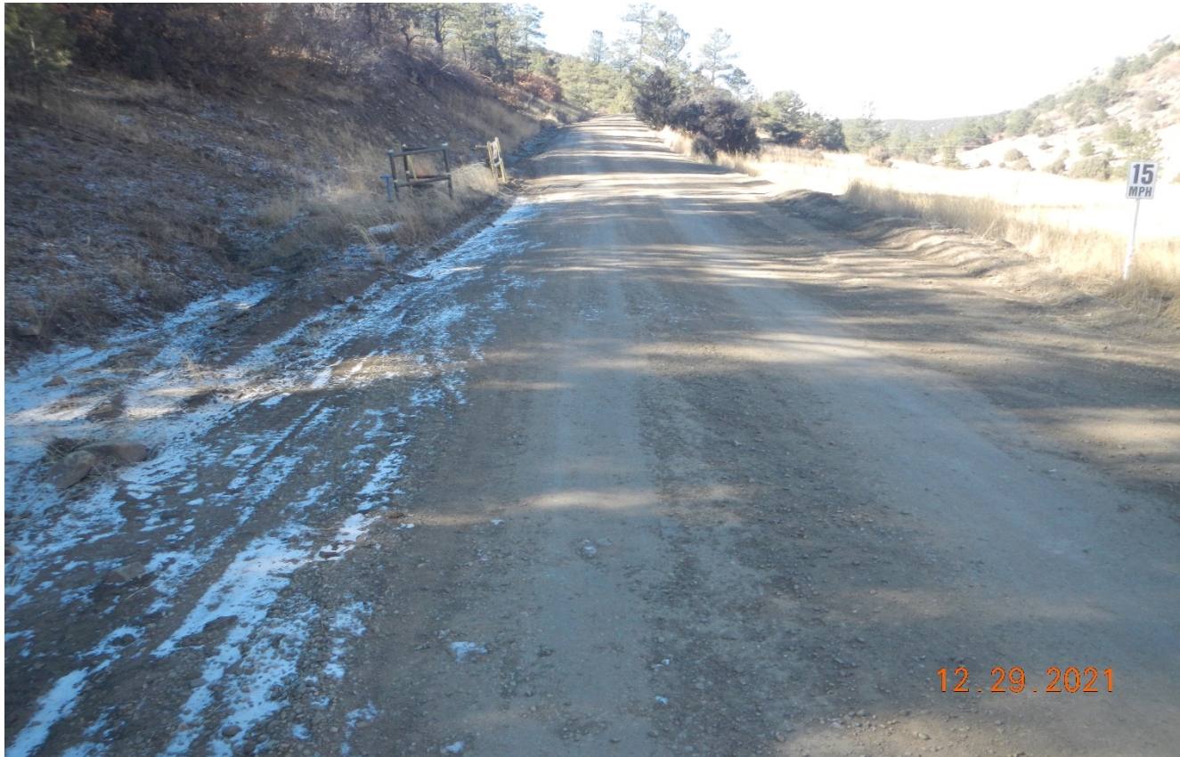
Photo 1. Facing southwest at the beginning of the road. The road has been regraded and crowned with road base.
