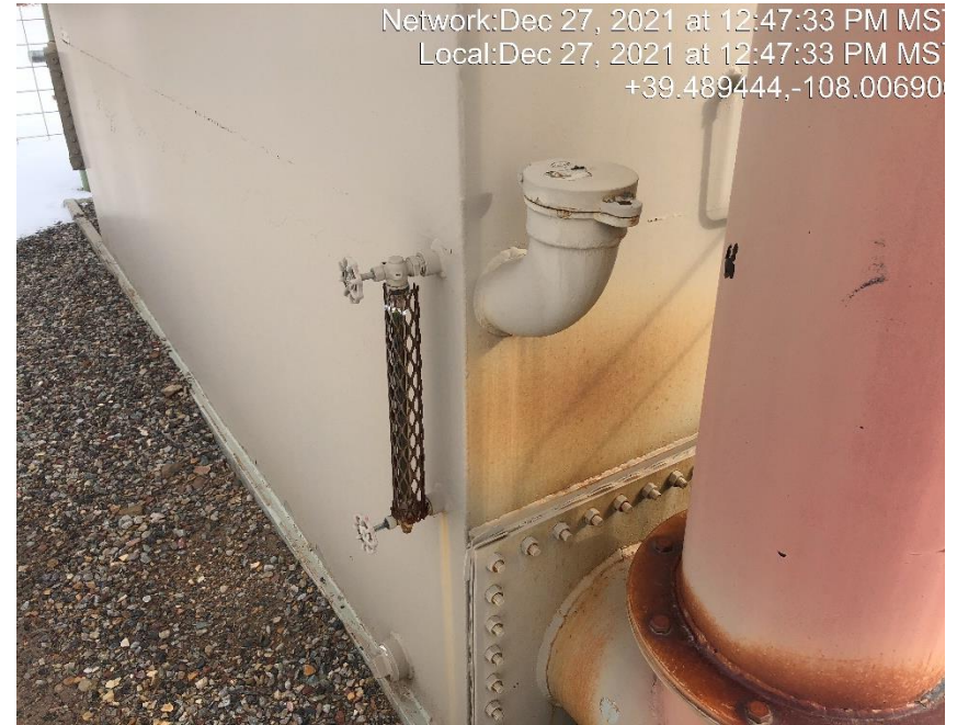
Photo #5510 Sight glass indicates the storage tank is full of an unknown fluid.
