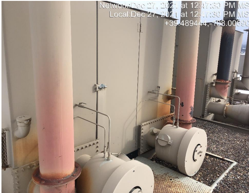
Photo #5509 Storage tanks not labeled.
