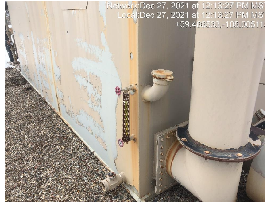
Photo #5506 Sight glass indicates that the storage tank is full of an unknown fluid.
