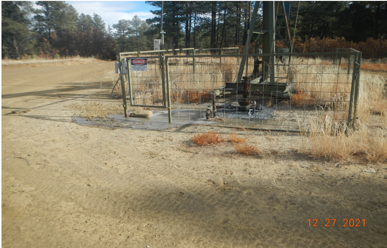
Photo 2. There is a dripping water leak at the wellheads that needs to be fixed.
