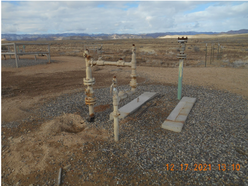
Separator risers locked out/tagged out
