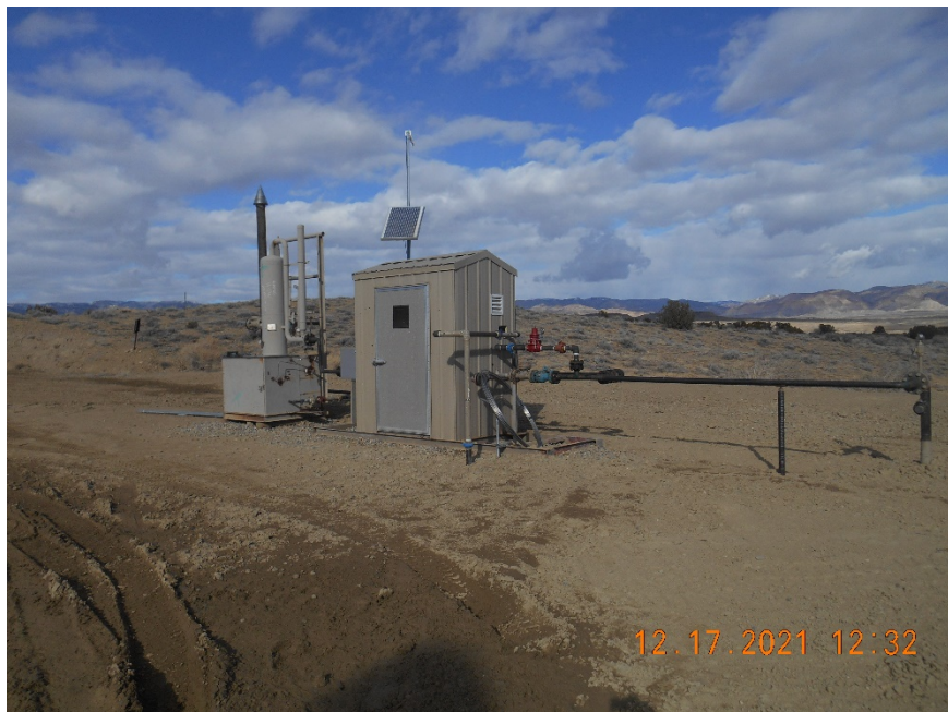
Separator with meter
