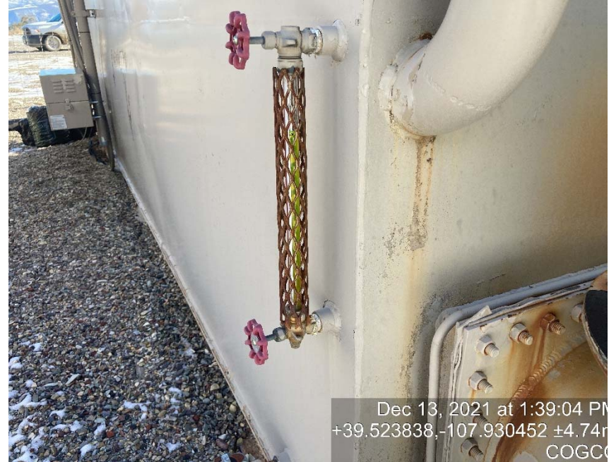
Sight glass shows fluid in storage tank
