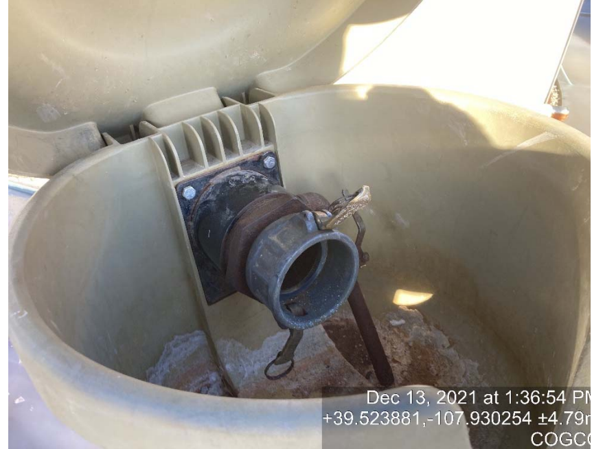
Load lines lacking bull plugs/caps
