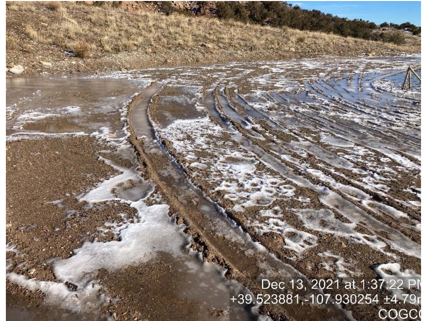
Lack of stabilization/compaction
