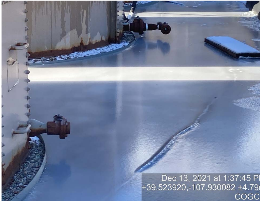
Load lines lacking bull plugs/caps
