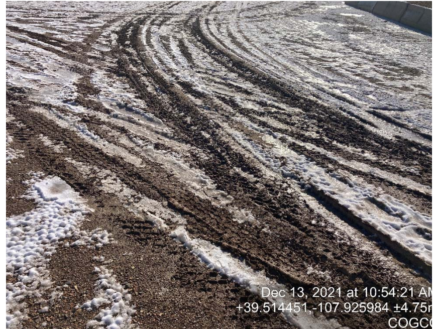
Lack of stabilization/compaction
