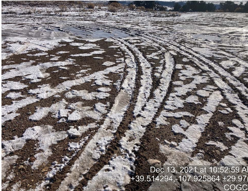
Lack of stabilization/compaction
