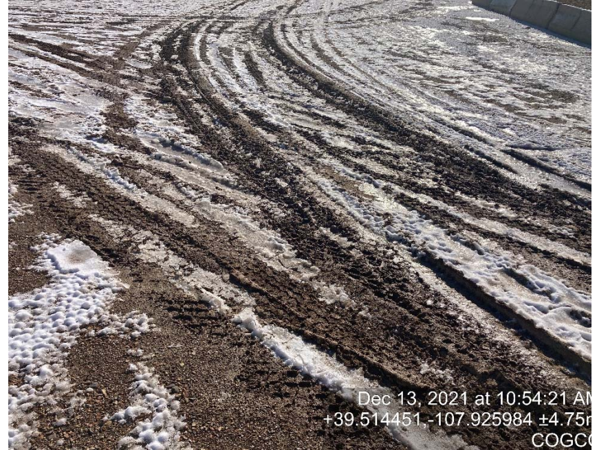
Lack of stabilization/compaction
