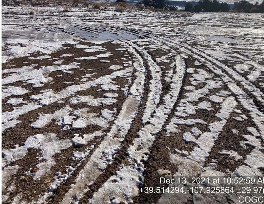
Lack of stabilization/compaction
