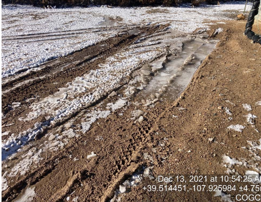
Lack of stabilization/compaction
