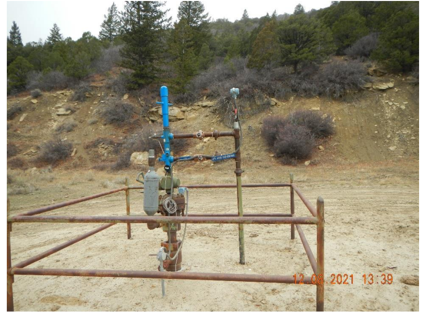
API# added to well signage.
