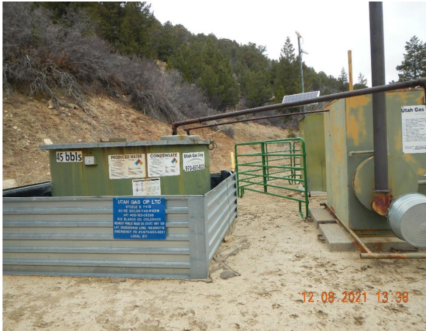
Sign installed at tank battery.
