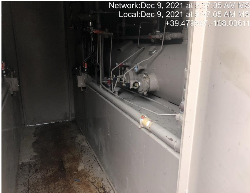
Photo #5375 Storage tank located under Horizontal separator.
