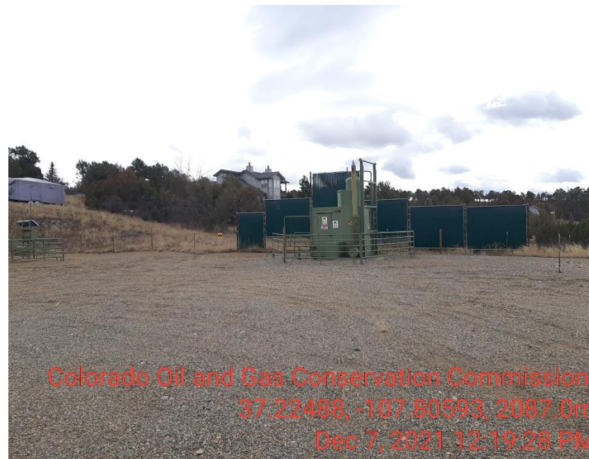
Photo 4 Vert sep and meter run
