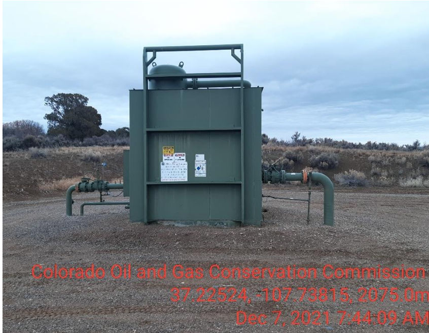
Photo 1 Sep/ meter run
