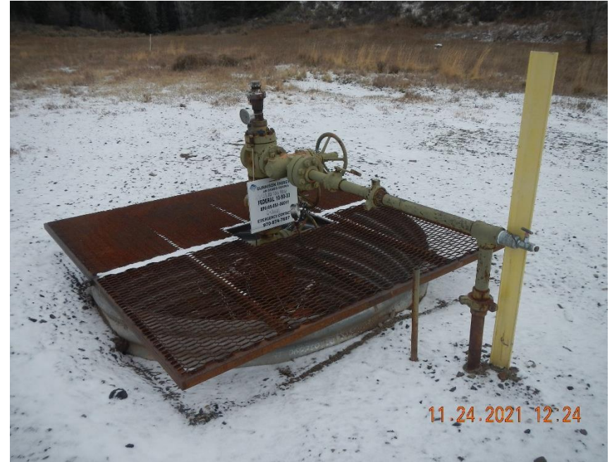
Federal 10-90-33 well head.
