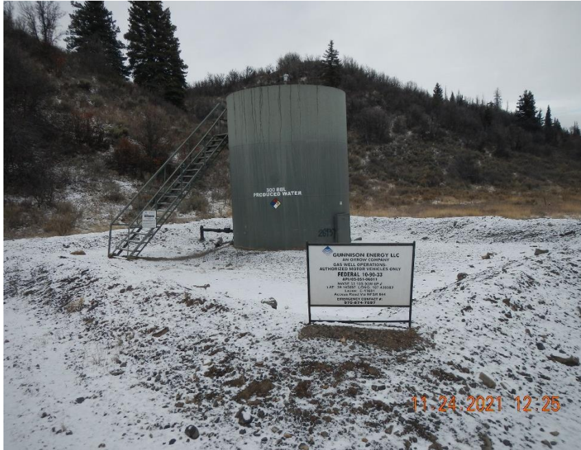
Federal 10-90-33 produced water AST.
