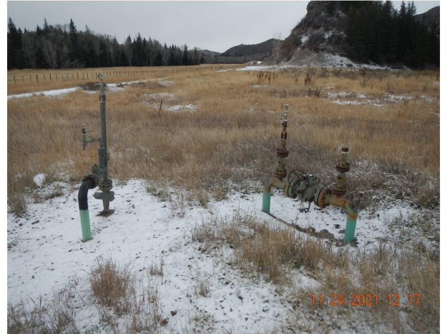
Off location flow line risers.
