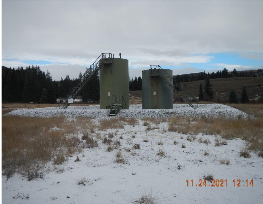
Federal 10-90-34 tank battery.
