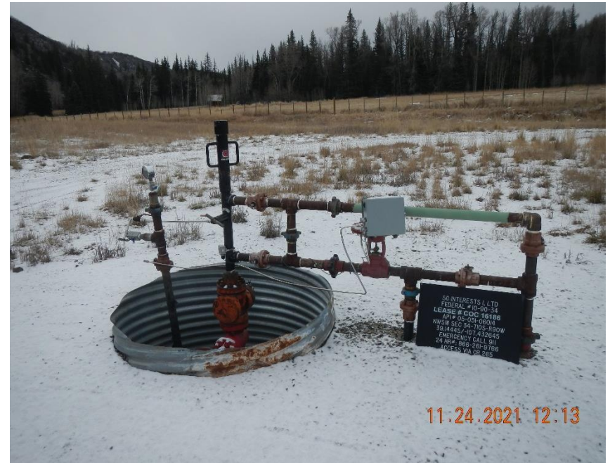
Federal 10-90-34 well head.
