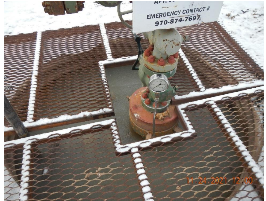
Cellar is full of ice. Expanded metal cover for cellar.
