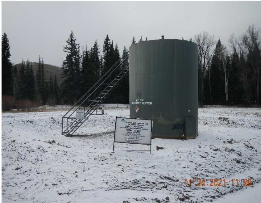
Federal 10-90-32 produced water AST with earthen berm.
