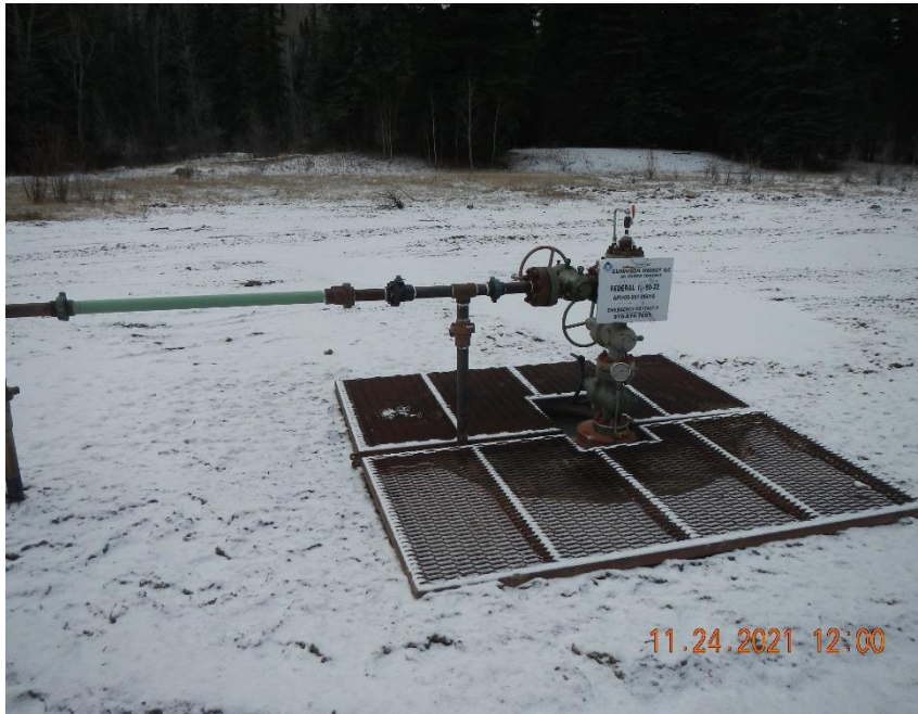
Federal 10-90-32 well head.
