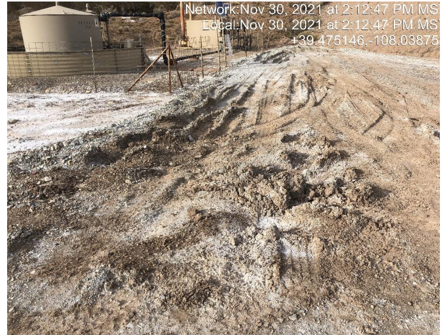
Photo #5296 Location lacks stabilization.
