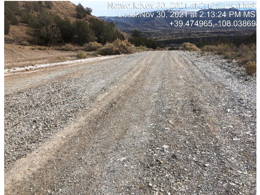
Photo #5298 Insufficient tracking control at entrance to location.
