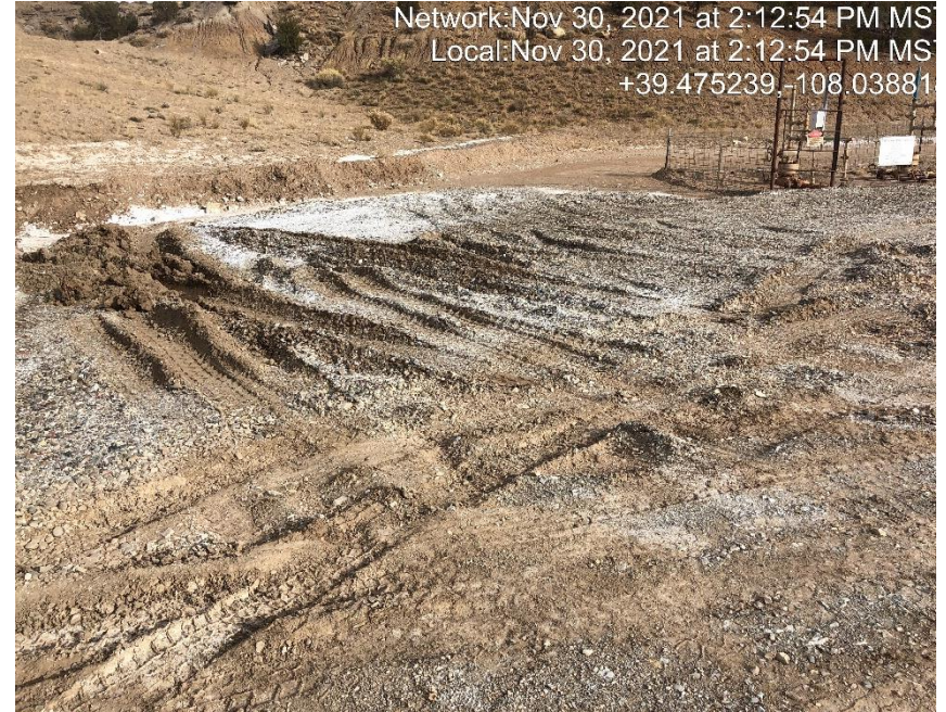
Photo #5297 Location lacks stabilization.
