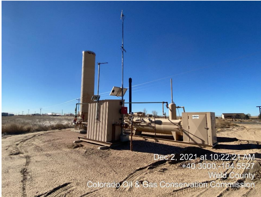
Photo #1 Production Equipment
