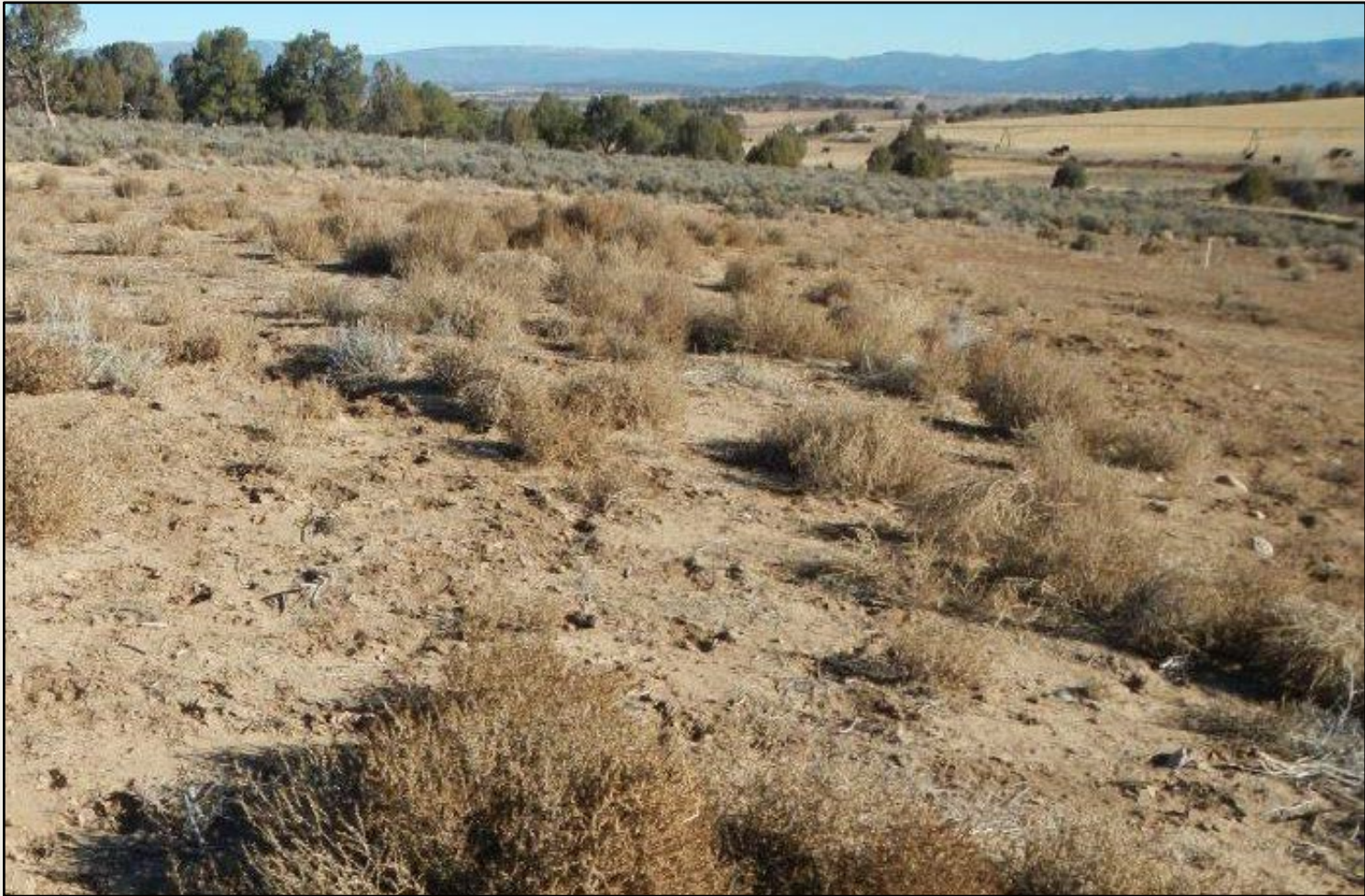
Photo 3. View of area within the southern fill slope with poor vegetative cover and dense Russian thistle.
