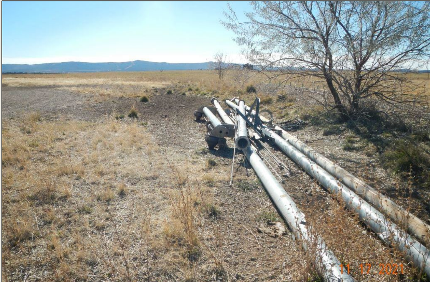
Photo 3. View of pipes within the western project area need to be removed.
