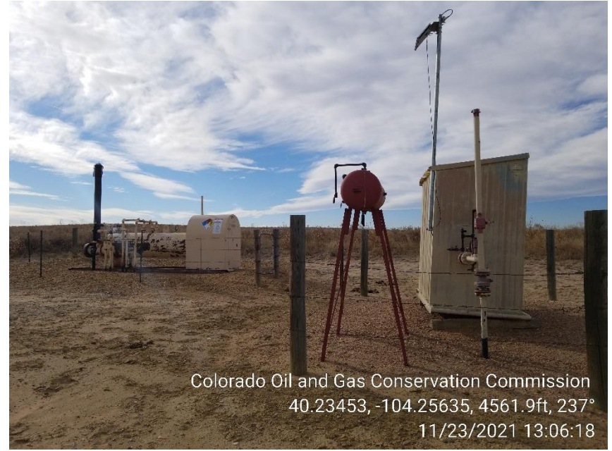
Photo 2 – Separator and Gas Meter
