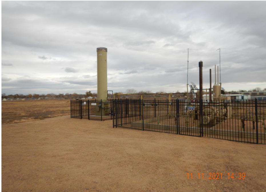
Photo 2. Photo taken from the associated tank battery, facing East. Photo illustrates the tank battery is still in use for other active wells.
