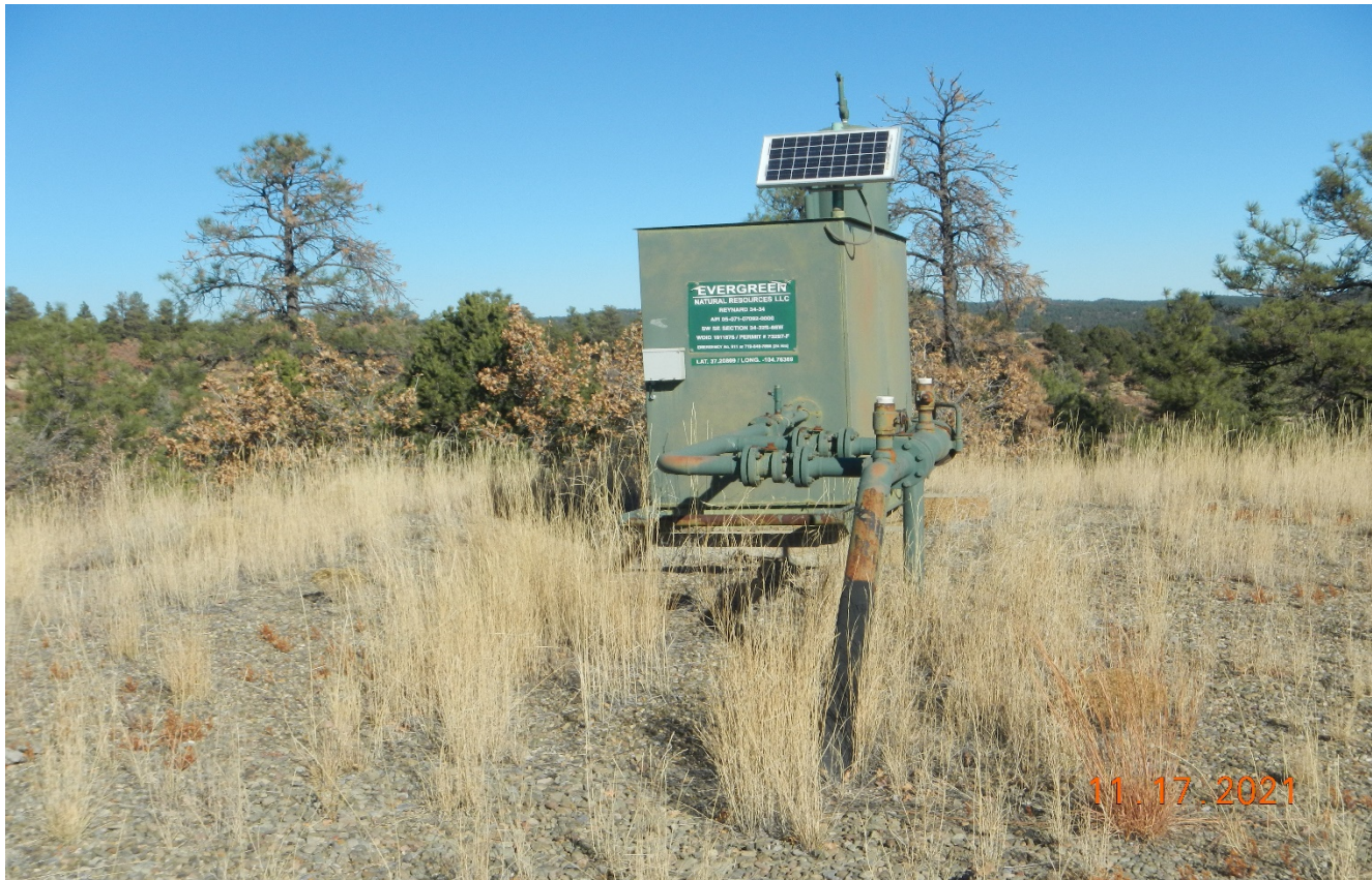
Photo 2. Well sign is posted.
