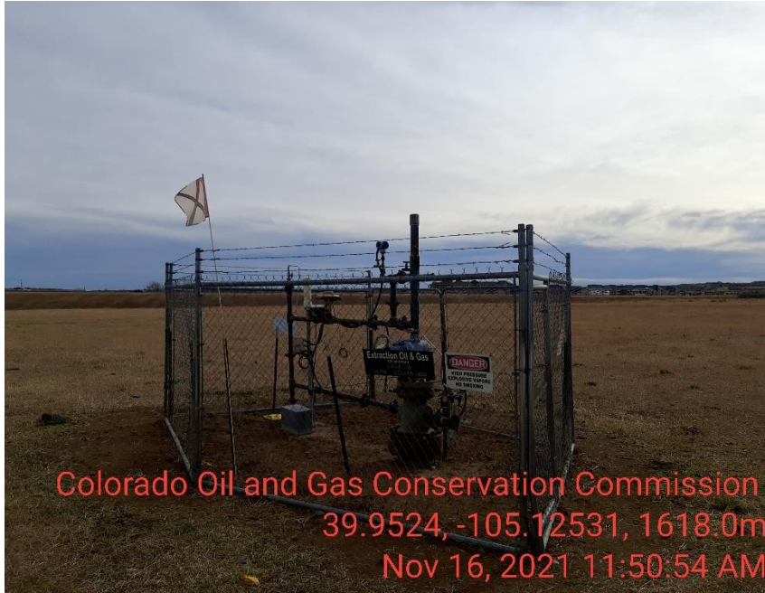
Photo 1 Well head is LOTO
