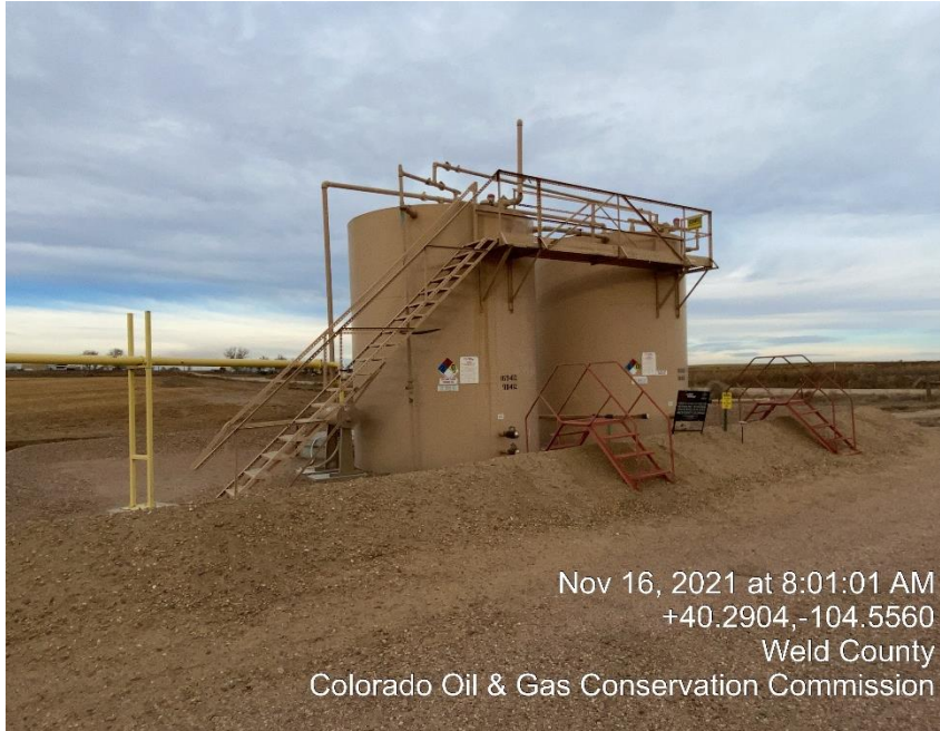
Photo #1 Tank Battery
