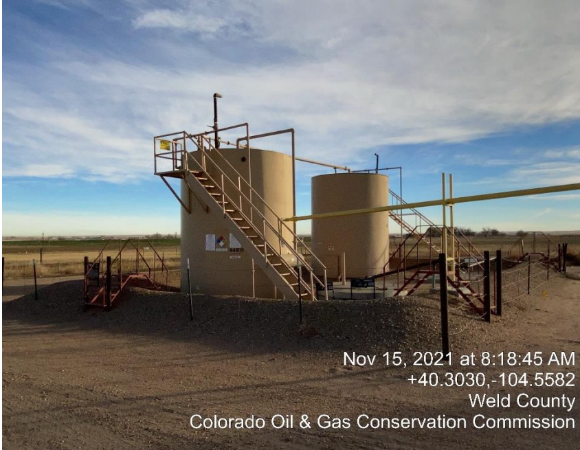
Photo #1 Tank Battery
