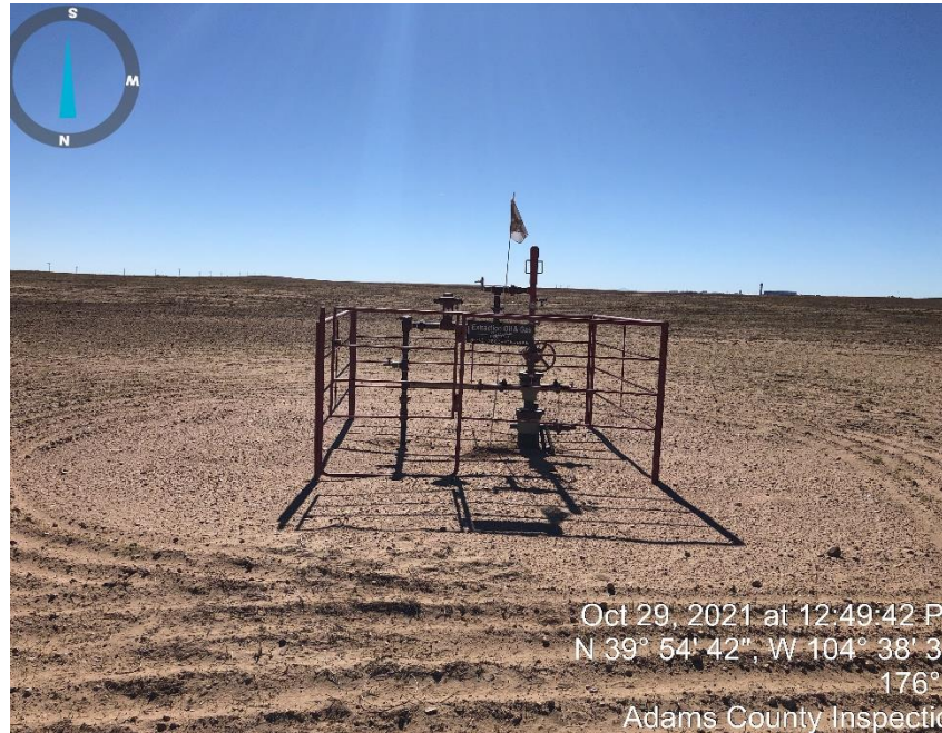
Photo #3 Well Head.
