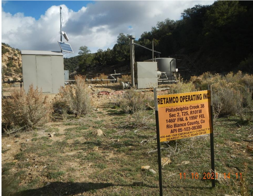
Tank battery sign not at tank battery.
