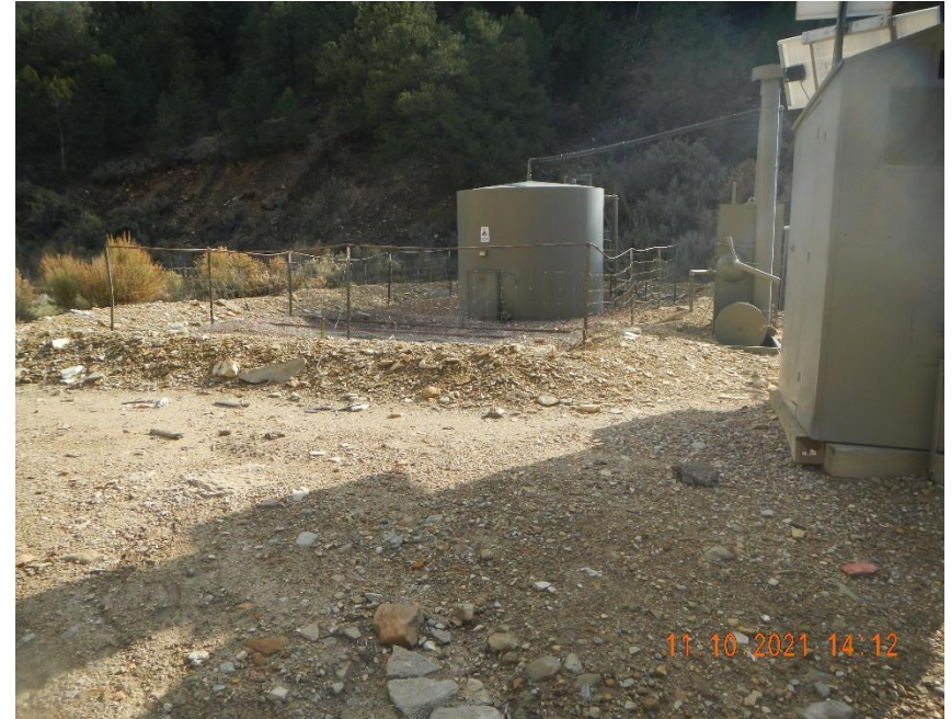
Tank battery sign not at tank battery.
