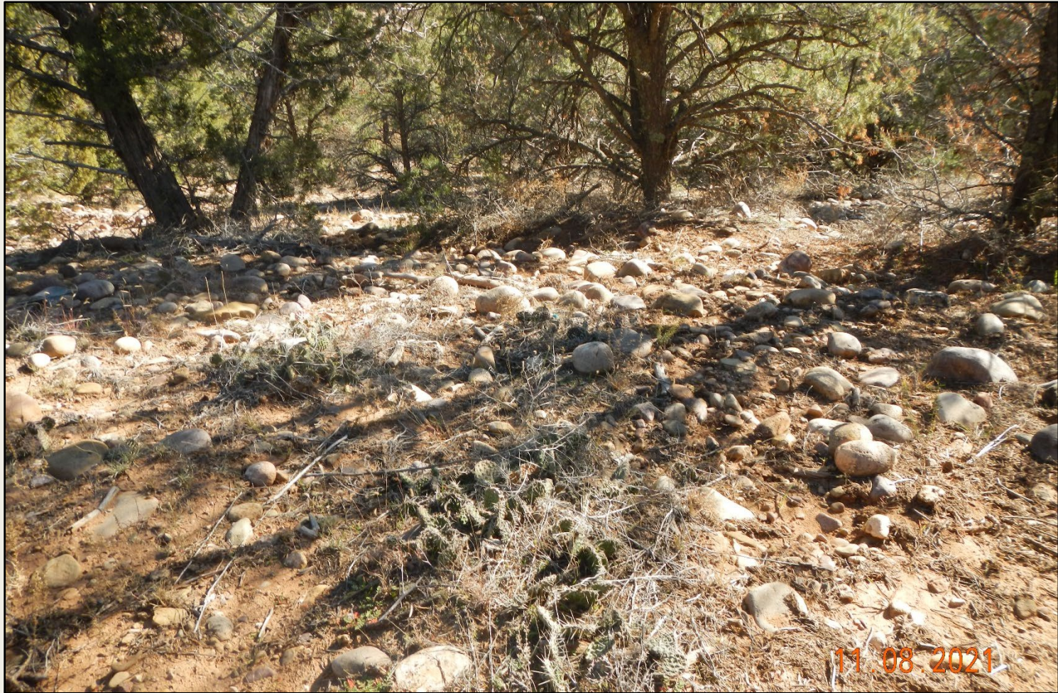
Photo 5. View of flood channel in the northern project area; gravel removed and wattles installed. Banks are not stabilized. Reseeding and stabilization not conducted. Wattle is not an appropriate stormwater control for this area.
