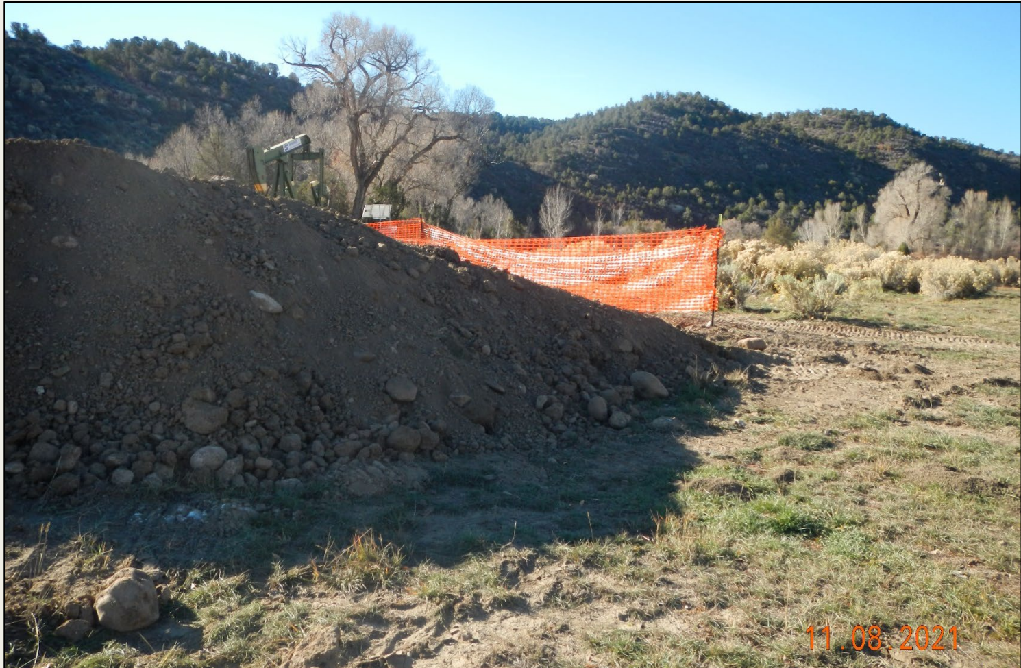
Photo 3. View of the northern project area from the northeastern corner facing westward. Flowline excavation is occurring in the northern project area.
