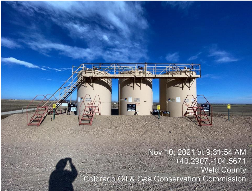
Photo #1 Tank Battery
